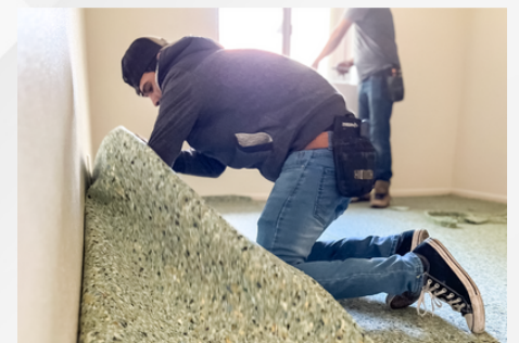
Professional installation of their premium RMX carpet, vinyl plank, and sheet vinyl options are among the core services RM Interiors provides.
